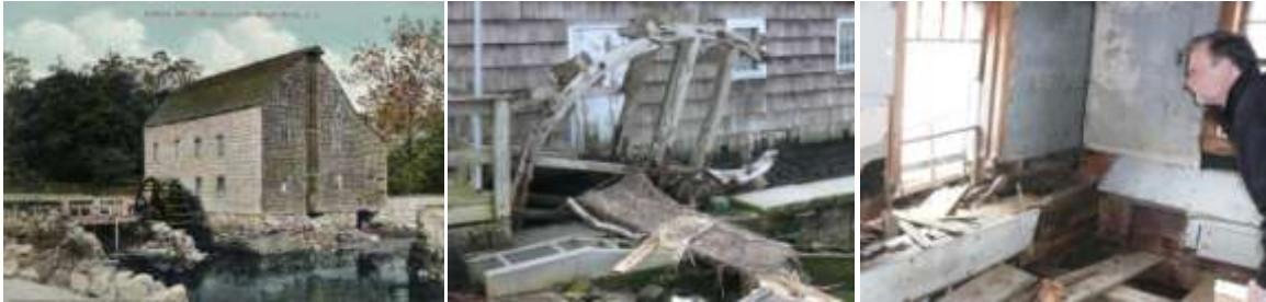
[L] Saddle Rock in better days. [C] The wheel has deteriorated. [R] Architect views winter storm damage.
